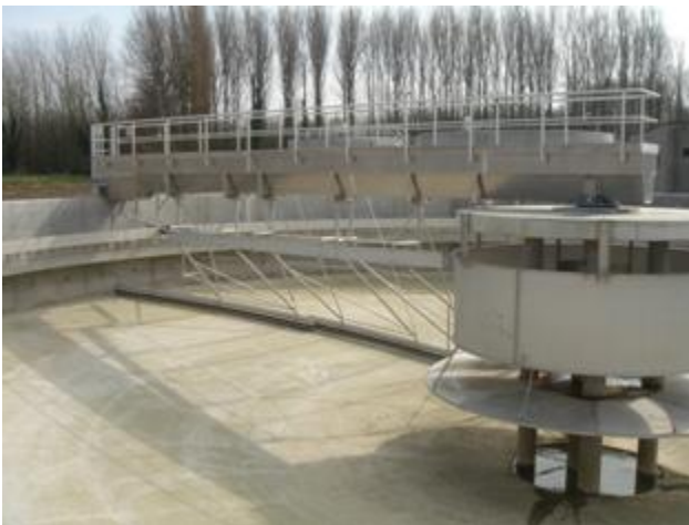
Empty sedimentation tank at the treatment plant in Merchtem
