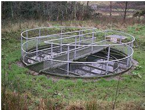
Secondary Sedimentation tank at a rural treatment plant
